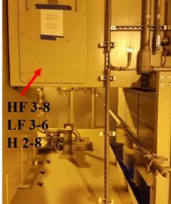
Photo 5: Generator Connection Box Sniffer Results.
