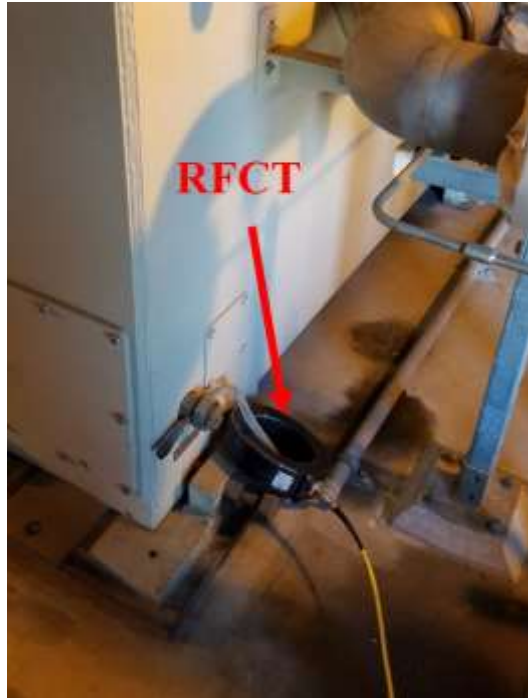
Photo 1: RFCT location for Generator.
